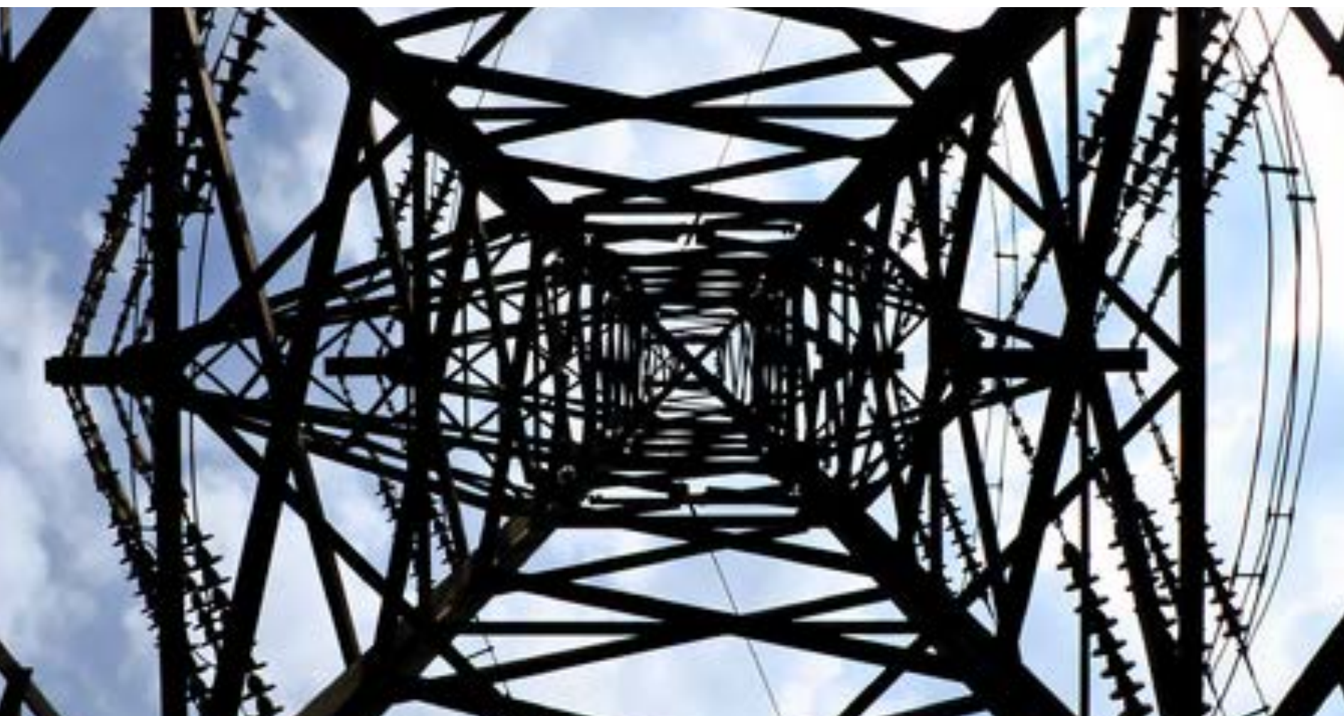
Steel utility tower
