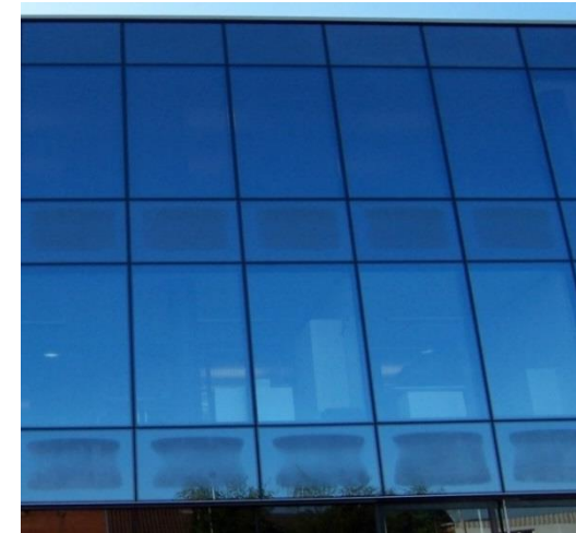
Condensation on external glass of spandrel boxes
