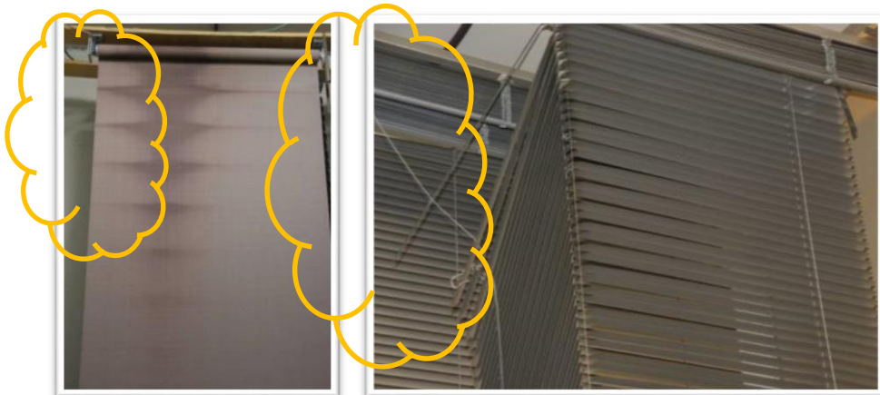
Single component failure of shading
