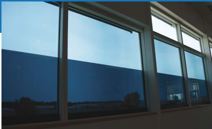
FIG. 4: EXAMPLE OF IN-PANE ZONING OF EC GLASS, WHICH IS NECESSARY TO APPROPRIATELY BALANCE THE COMPETING NEEDS OF GLARE CONTROL, DAYLIGHT ADMISSION, ENERGY PERFORMANCE, AND LIGHT COLOR QUALITY.
